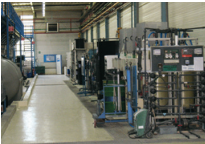
< Legrand has been involved in the reduction of the environmental impacts of its sites for many years, as in the Altis production plant: paint effluent treatment plant
